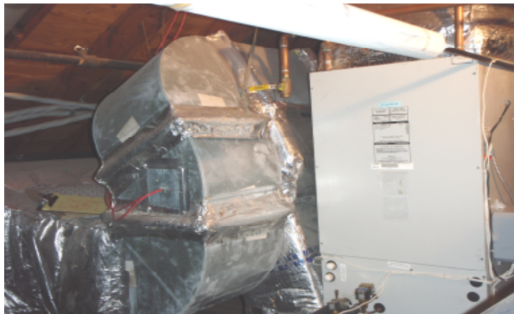
Ductwork Connection to Dehumidifier
